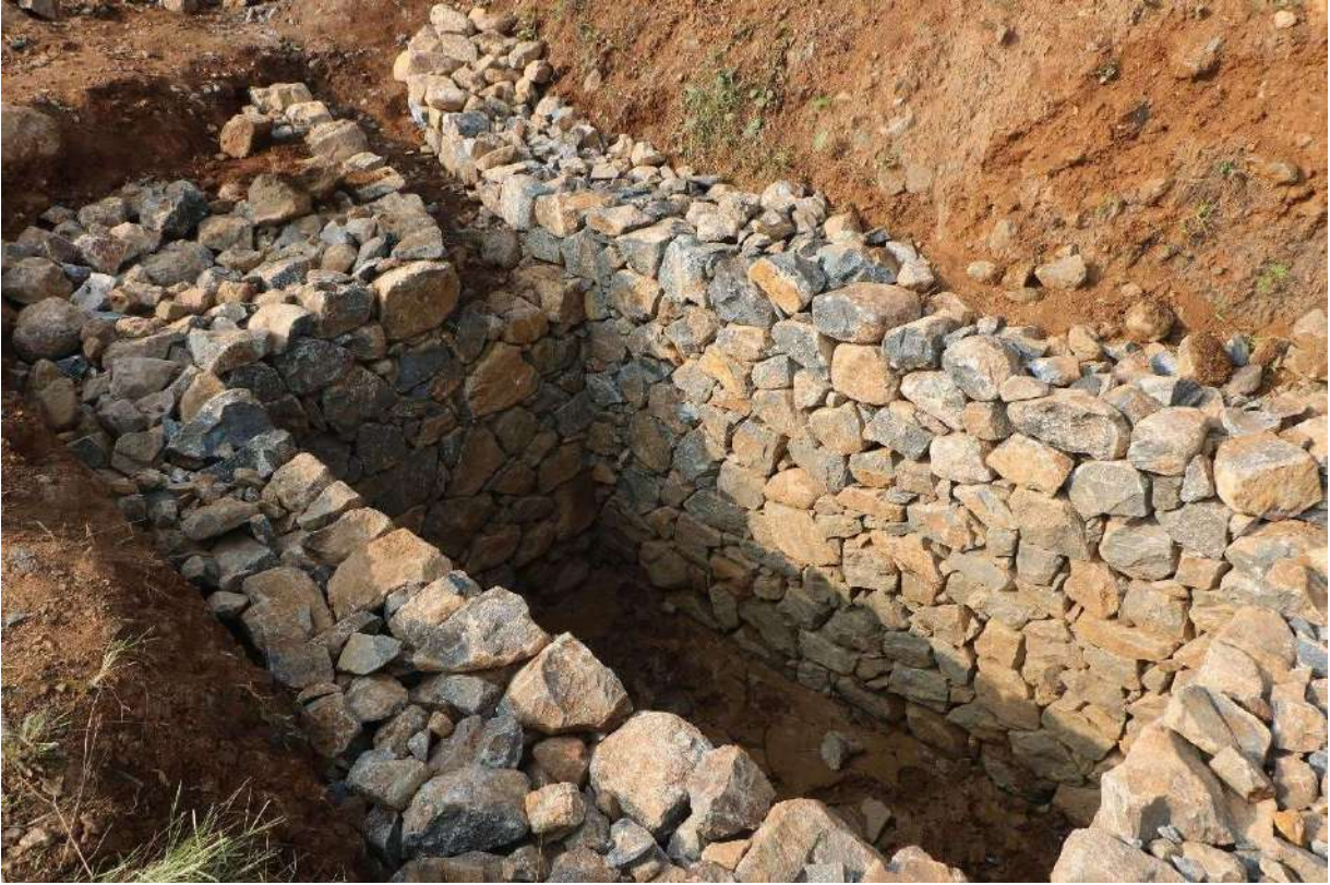
Settling tank for the overflowing water
